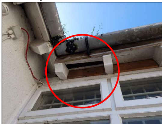
Figure 9 – Closer View of Damage to Wooden Soffit Recorded at Rear (E) Side of Building
