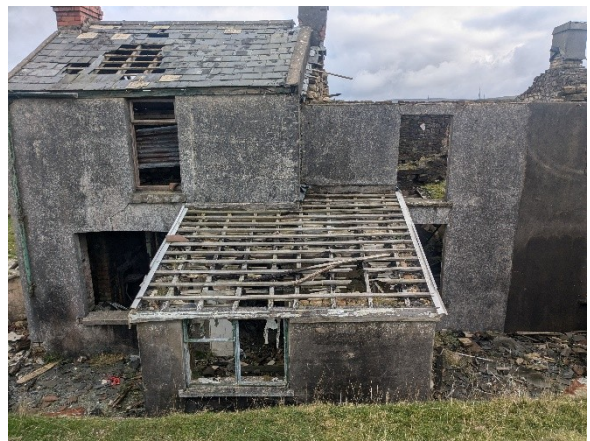
Multiple PRFs identified behind timbers, beneath roofing materials and within chimneys.
