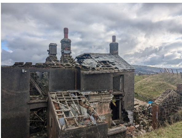
Multiple PRFs identified behind timbers, beneath roofing materials and within chimneys.
