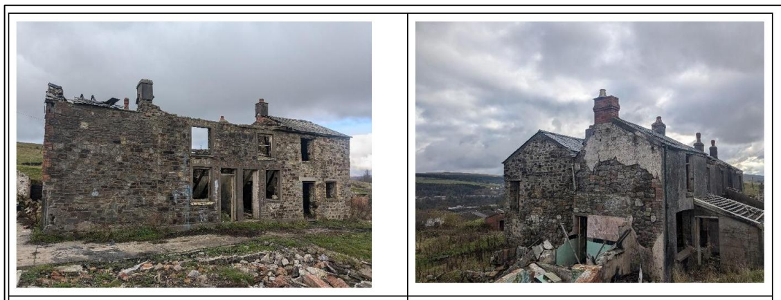
Photographs 9 & 10 – Showing the remains of the former farmhouse at the site
