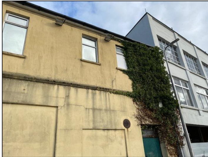
Photo 15 – evidence of window openings of different heights and cill levels
