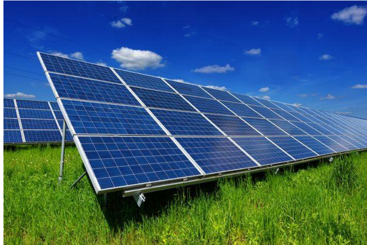
Figure 13 – Typical solar array appearance
