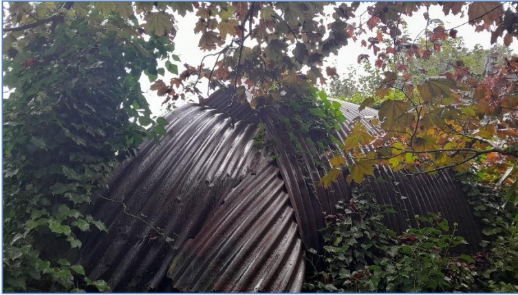
Photograph 9. The collapsing metal roof at the southern end on the Northern Section.
